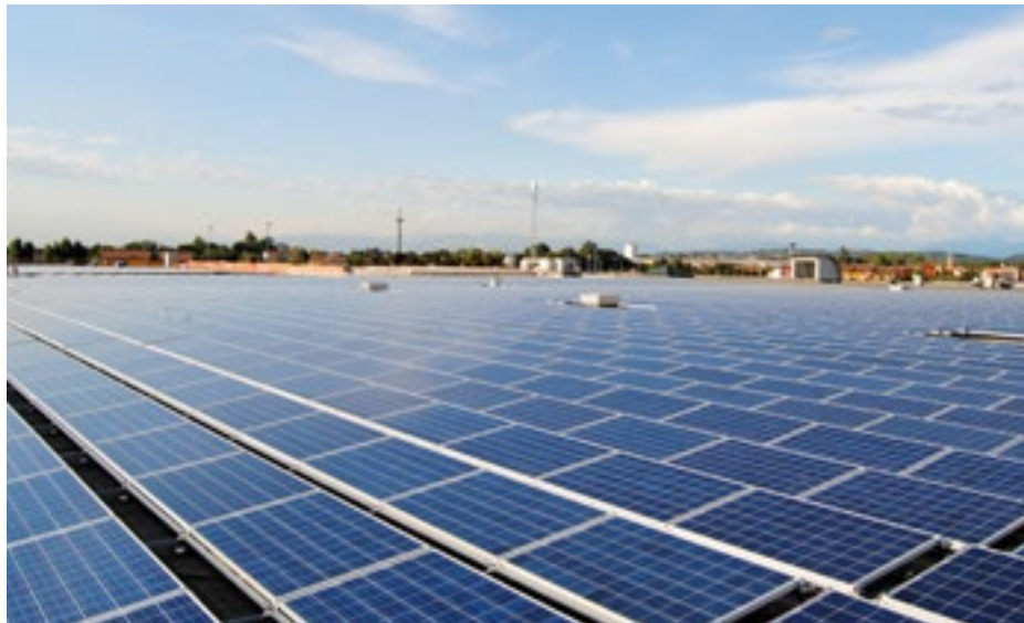
“Medole” Photovoltaic plant – 922 kW
